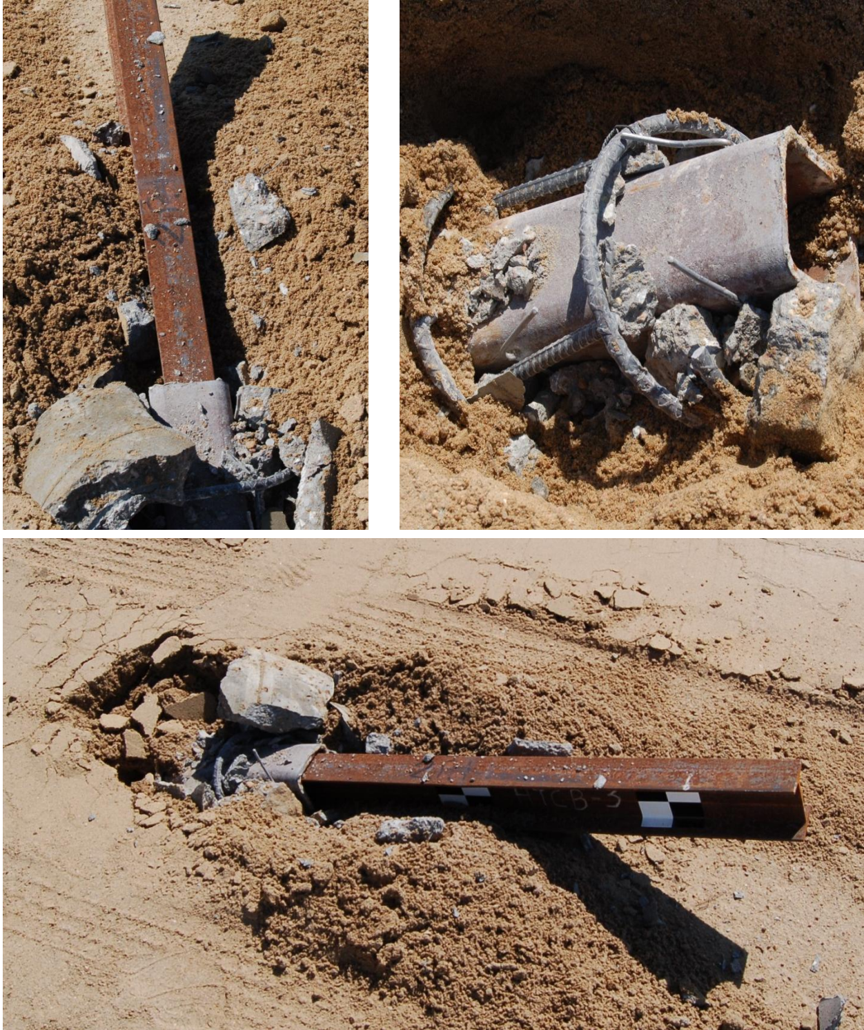
Figure 5.11 System Damage, Test No. HTC3-3
